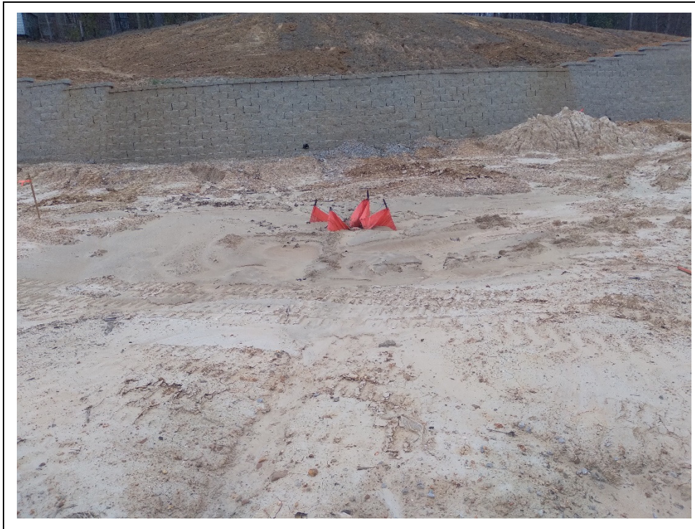
Photo #3: Temporary silt fence around inlet at the east side needs maintenance.
