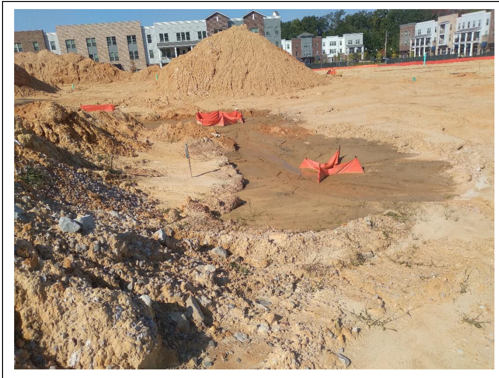
Photo #7: Several temporary inlets need to have silt removed
