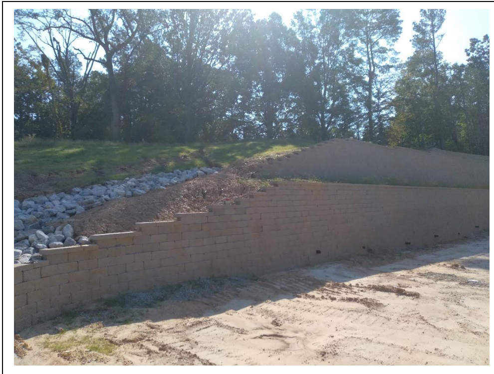
Photo #5: Wall #1, #4 and #5 looking east. Riprap and growing vegetation
