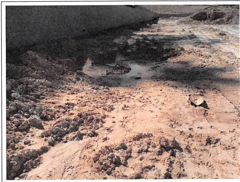
Photo #6: East side temporary inlet protection needs to be replaced
