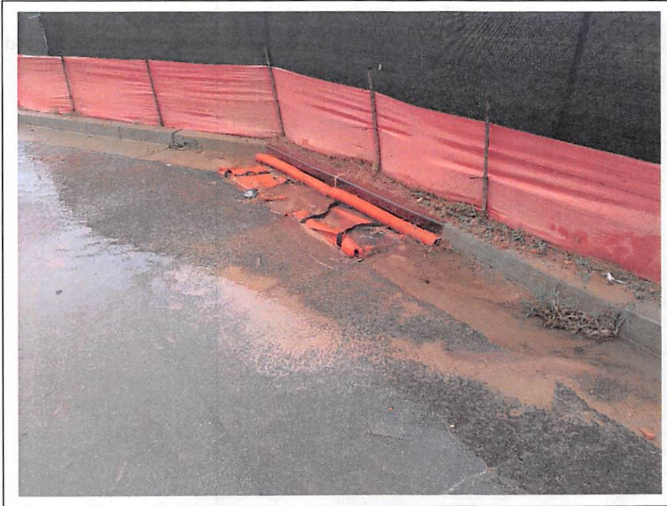
Photo #5: Inlet protection along Village Market Lane needs to have the silt bag replaced.
