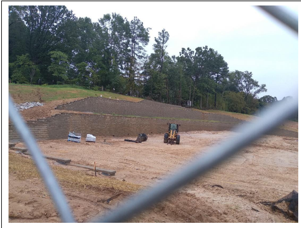
Photo #7: Vegetation growing behind Wall #1, #4 and #5 looking southeast.
