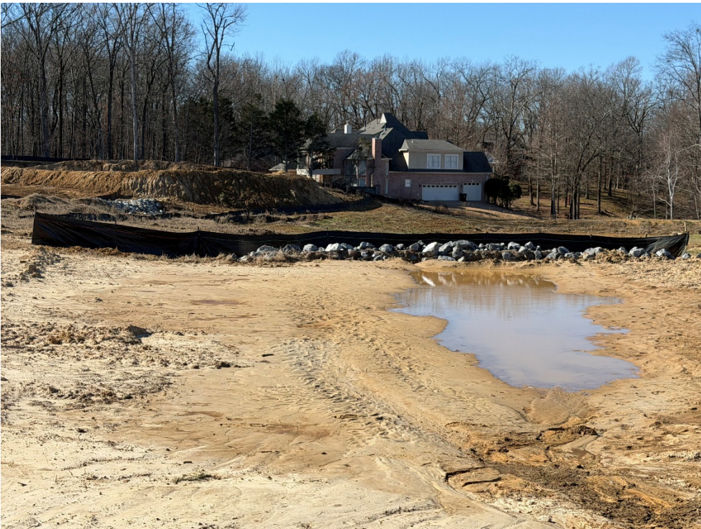
Photo 10: Silt Fence that has been installed for erosion control.
