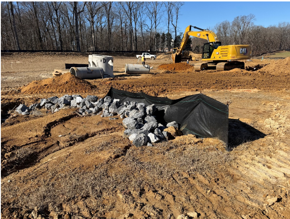
Photo 8: Silt Fence that has been installed for erosion control.
