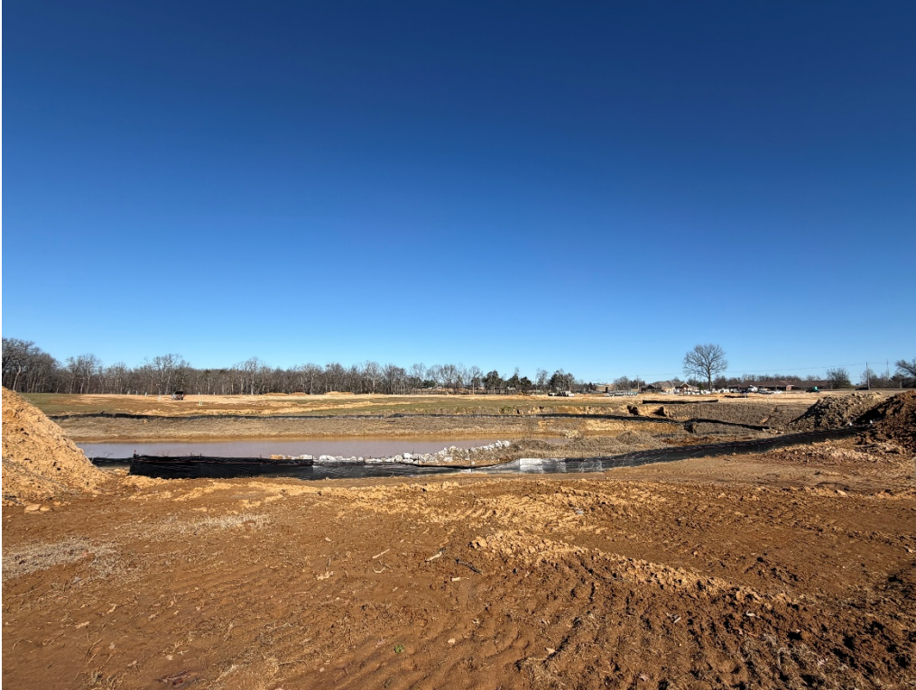
Photo 9: Silt Fence that has been installed for erosion control.
