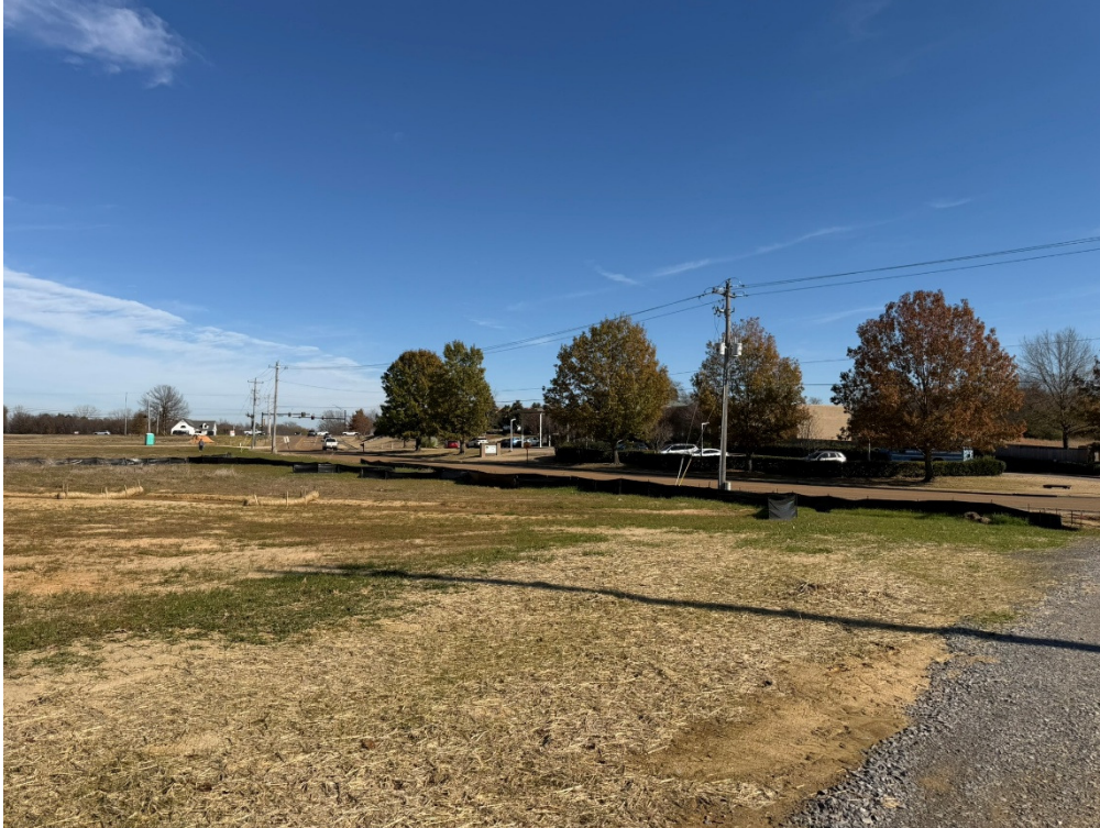
Photo 5: Additional Silt Fence was installed At the Lift Station Rd. and Davies Plantation Rd. to prevent erosion.
