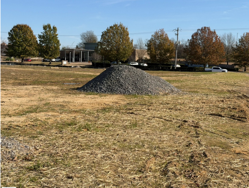
Photo 7: Additional Gravel that has been stockpiled, but will be used on the Lift Station Rd.
