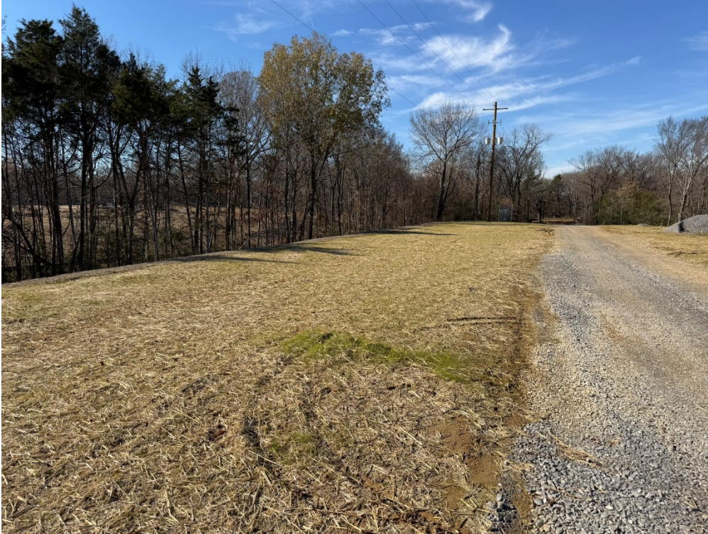
Photo 3: The slopes alongside the Lift Station Rd. have been temporarily seeded and mulched to prevent erosion.
