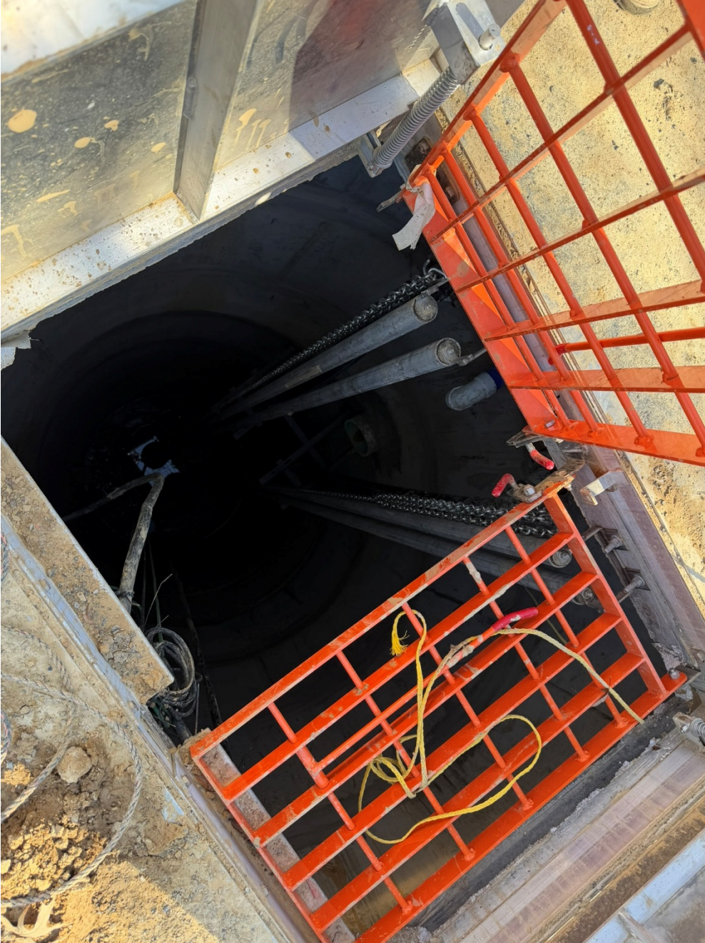
Photo 2: Equipment to raise and lower the pumps for service or repair has been installed at the Lift Station.
