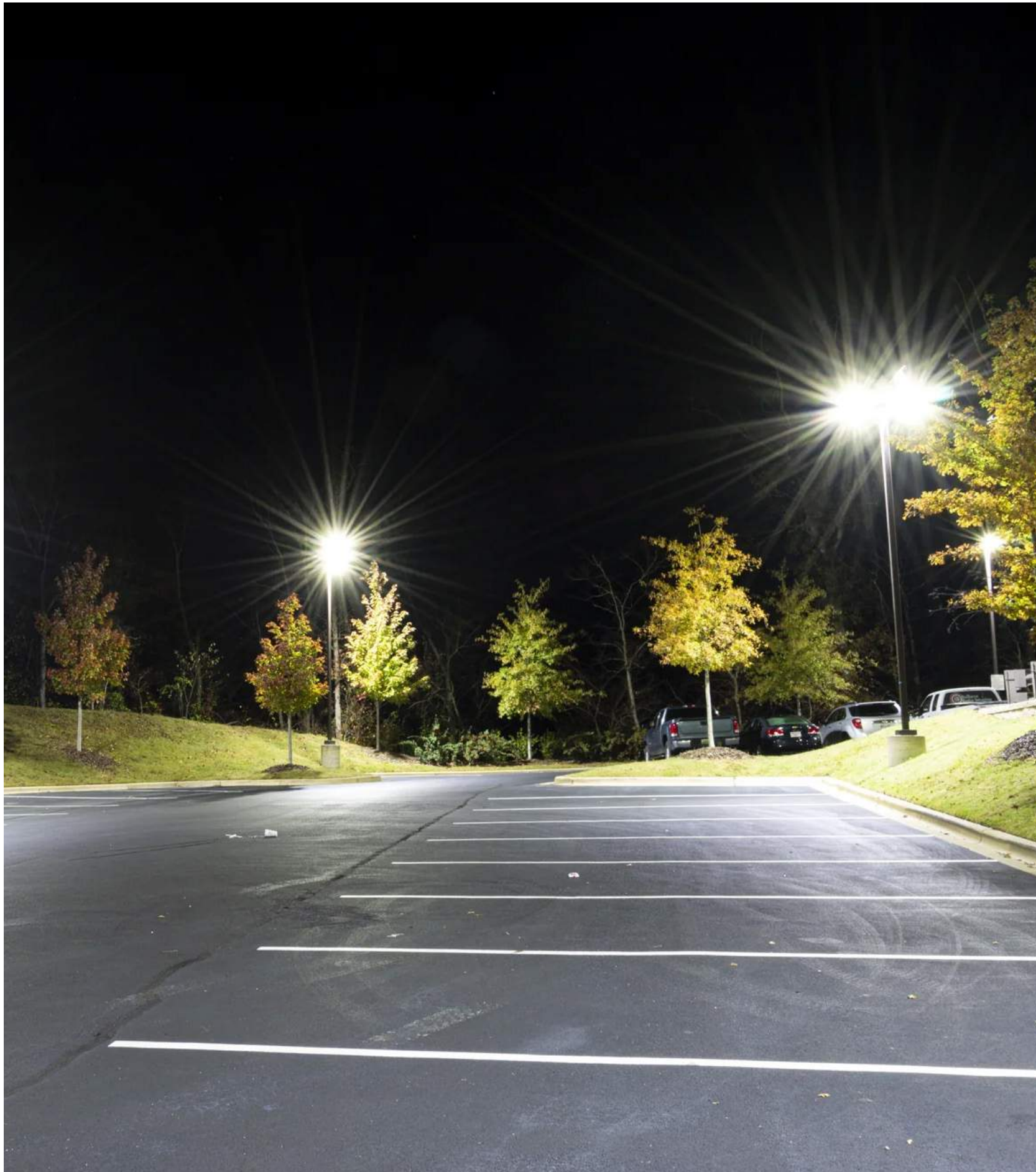
PARKING LOT LIGHTING
