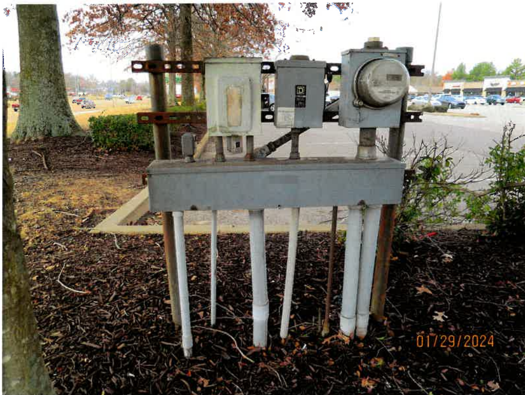
Electrical equipment for sign – to be relocated by contractor – excluded from valuation
