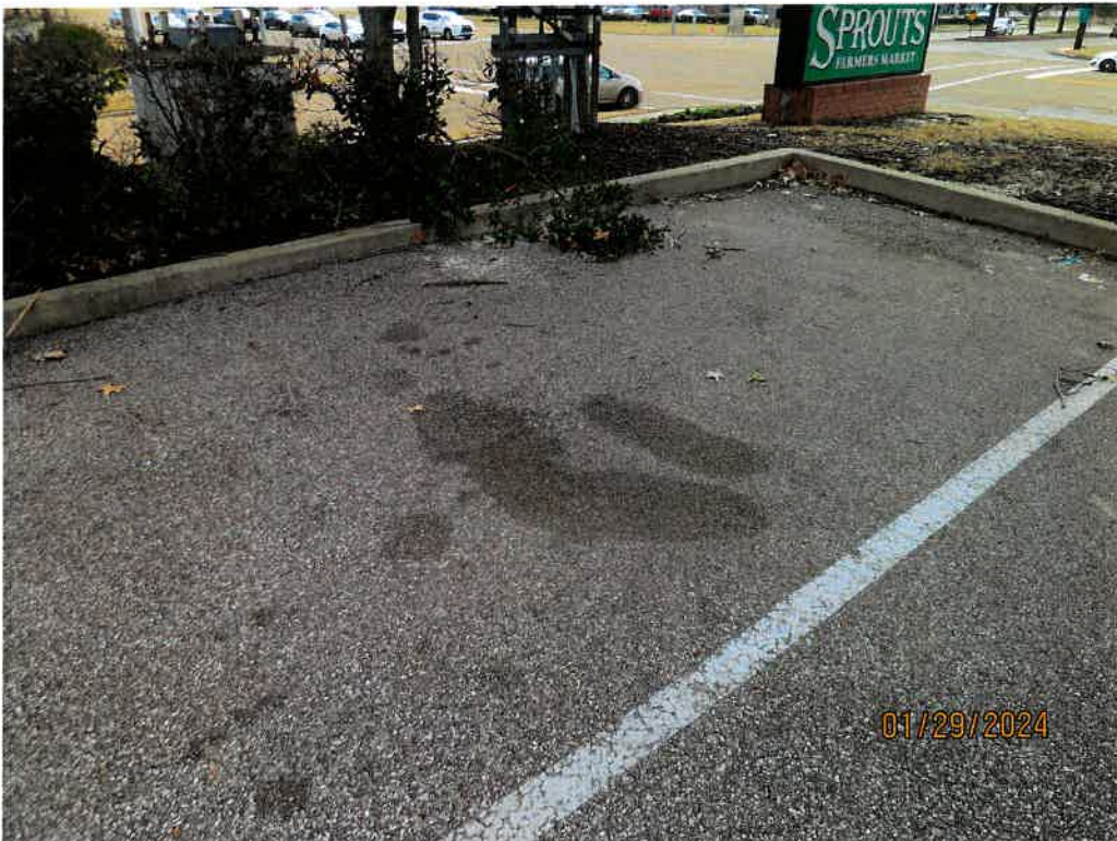
Improvement No. 4 – paved asphalt and lost parking spot
