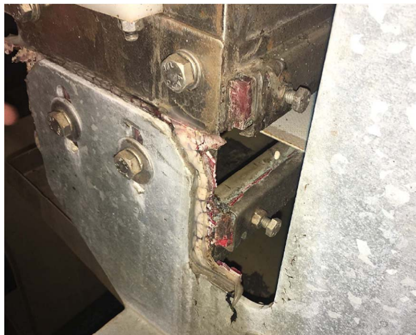
Wash boxes need rebuilt
