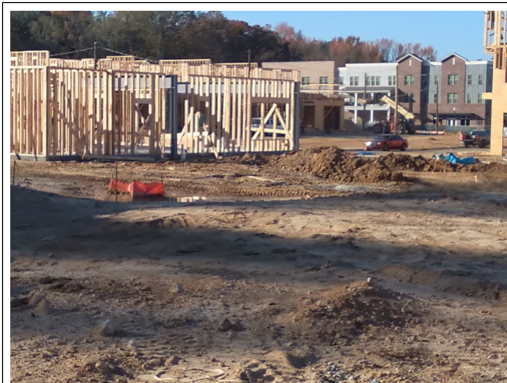
Photo #4 South end of site needs temporary inlet maintenance.
