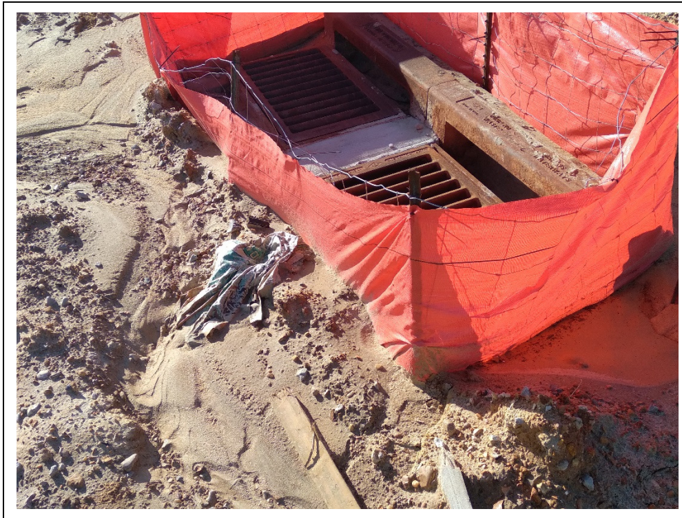
Photo #3: Temporary silt fence around permanent curb inlet needs to be maintained.
