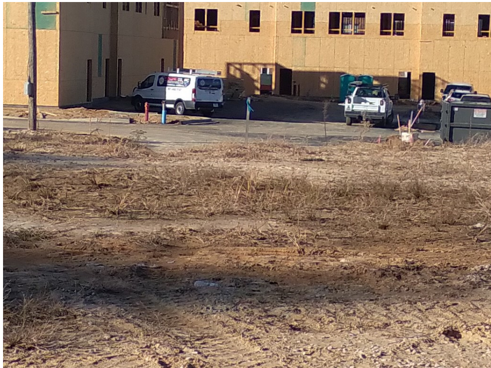
Photo #2: Post Indicator valve installed at west side of site.
